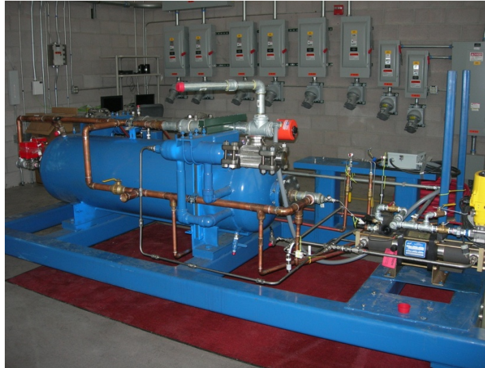
Figure 3-8: Brayton Cycle compression loop (In the process of re-assembly at Sandia National Laboratory)
