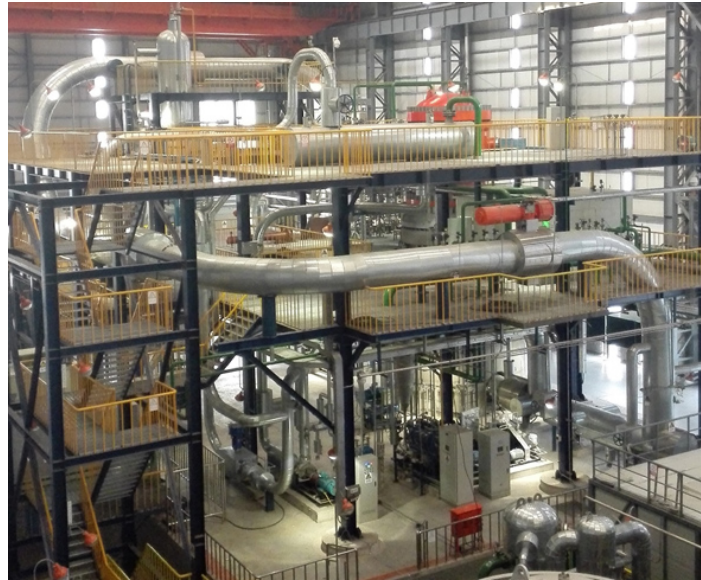
Figure 3.53: Engineering test facility of main helium circulator (ETF-HC) at INET's HTR-PM Laboratory
