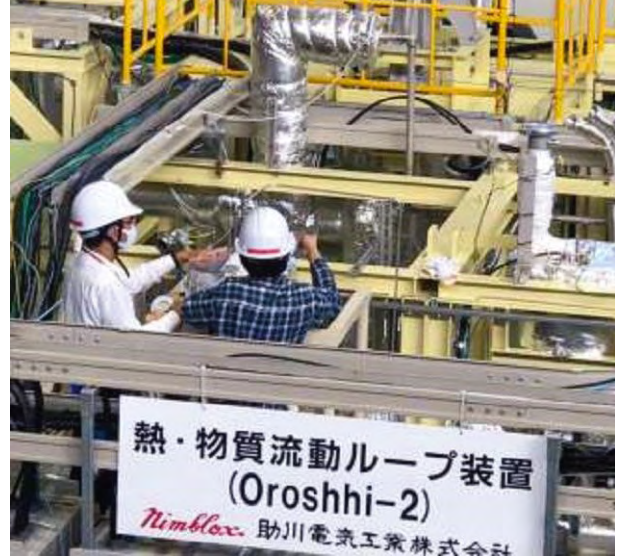
Figure MSR-9. FLiNaK molten salt loop at the National Institute for Fusion Science
