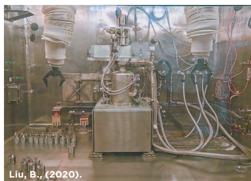
Figure VHTR-2. KÜFA furnace installed in INET hot cells
