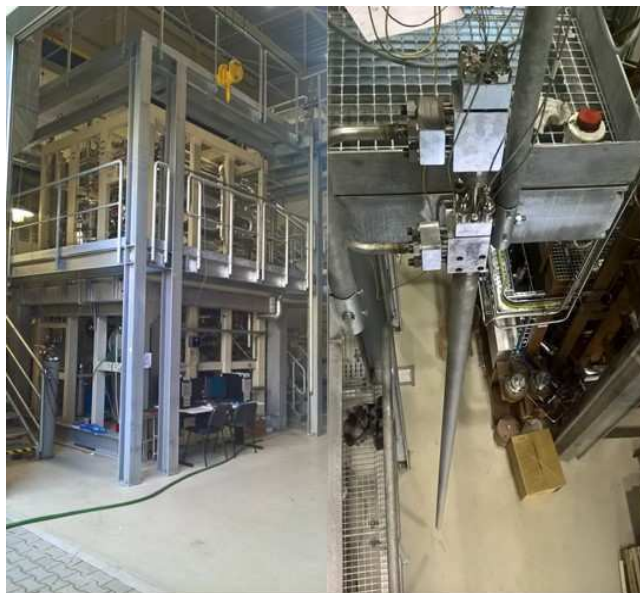
Figure VII-12: In-Reactor SCW Loop and Test Section at CVR in Czech Republic
