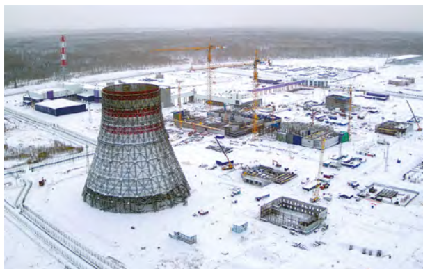
Figure LFR-2: Construction of the BREST-OD-300 power unit as part of the Pilot Demonstration Energy Complex
