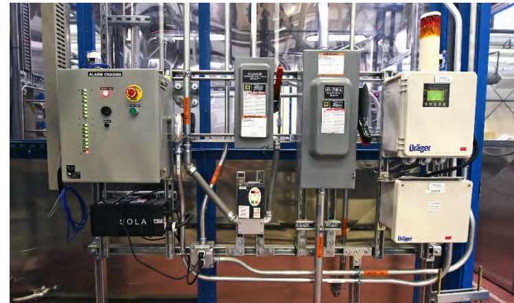
Gas alarm and Interlock System
