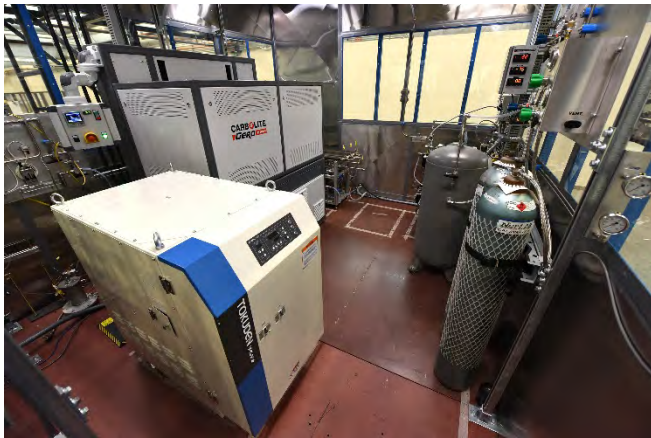
Enclosure Interior View
