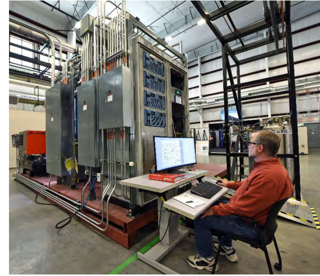
25 kW HTE Test Facility Control Station
