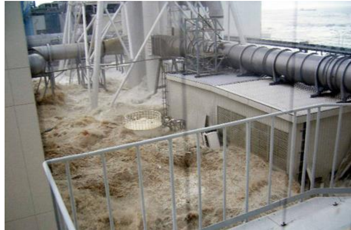
Backup diesel generator at Fukushima engulfed in water due to Tsunami Courtesy of TEPCO
